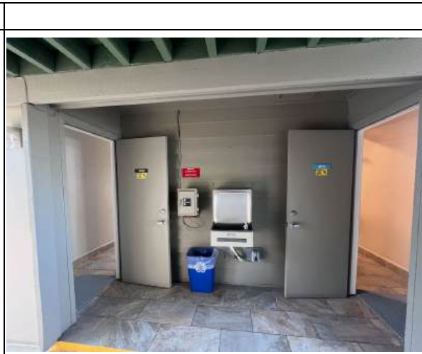
Pool Equipment Structure
