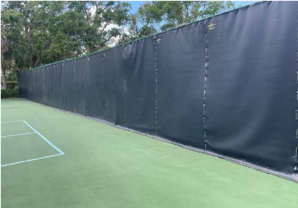
Pavilion Tennis Court Acoustical Panels
