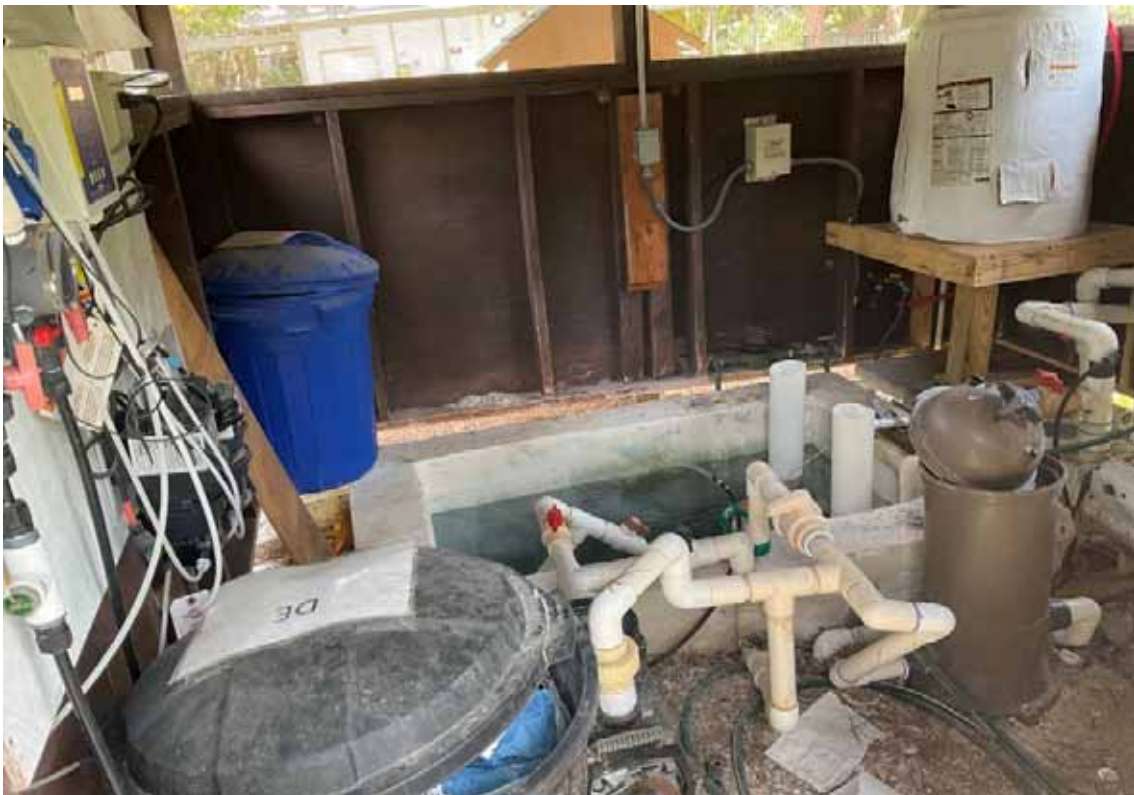
Glenhouse Pool Equipment
