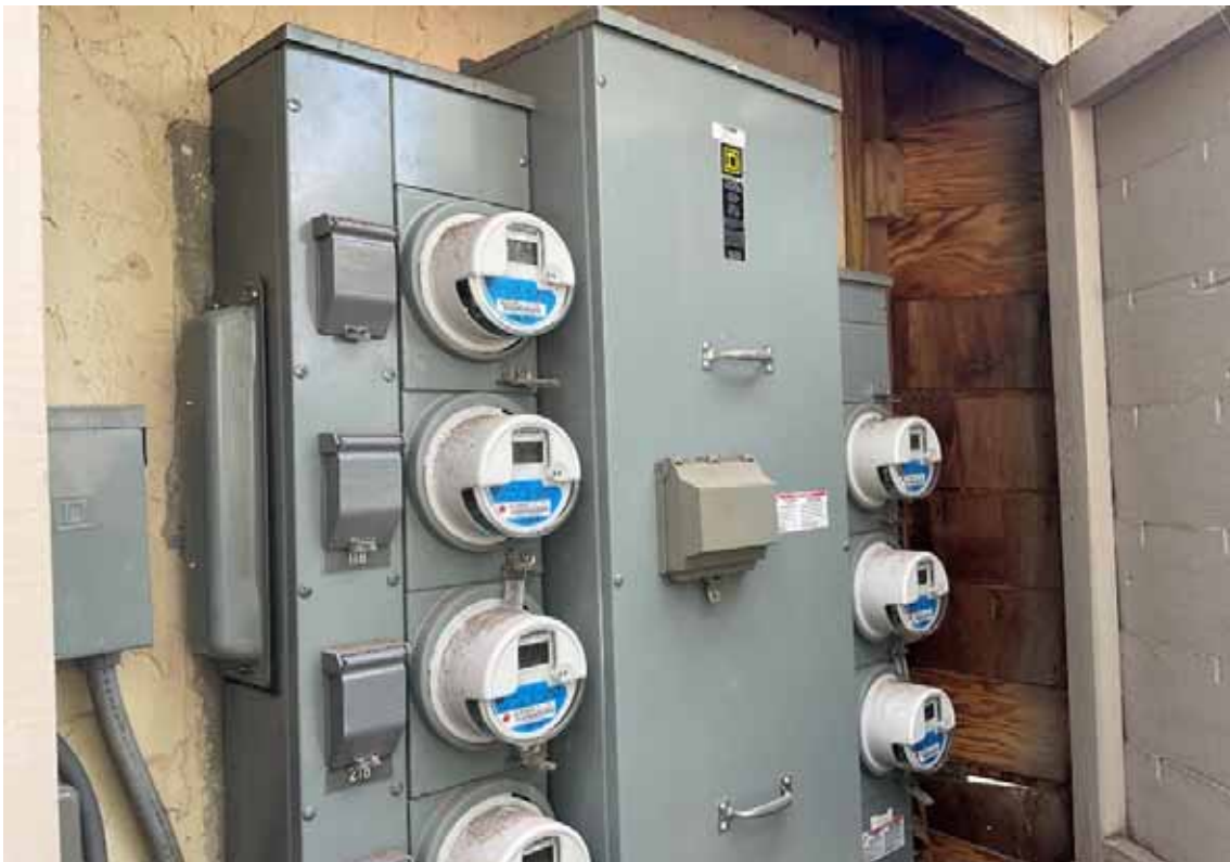
Condo Bldg Electrical Panel (New)
