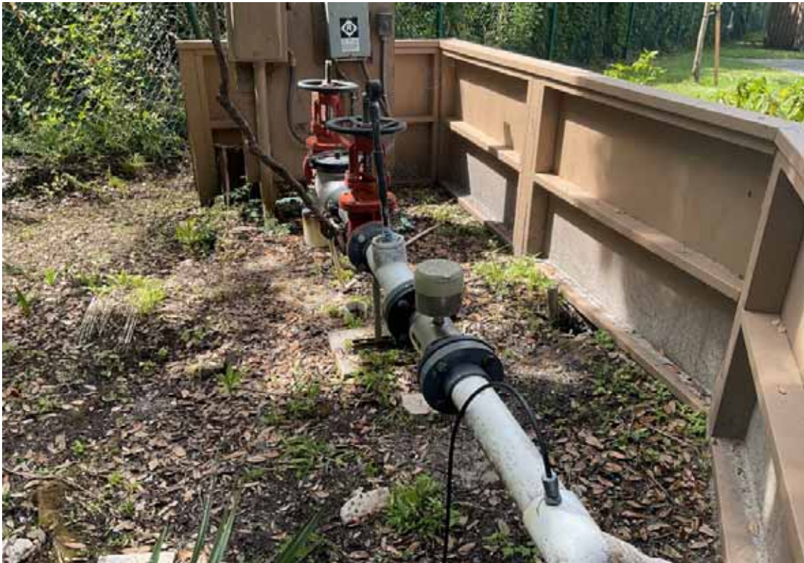
Well Pump - Brookhouse
