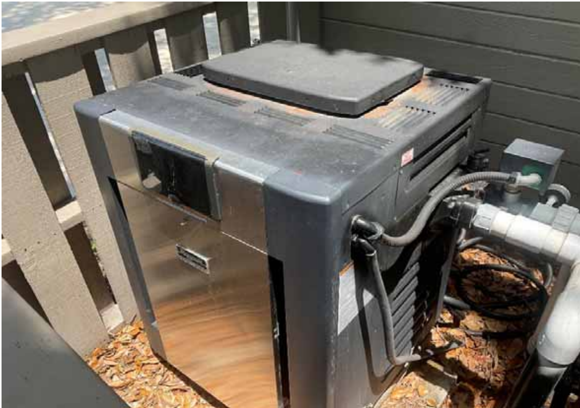
Harbor Club Pool Equipment, Heater
