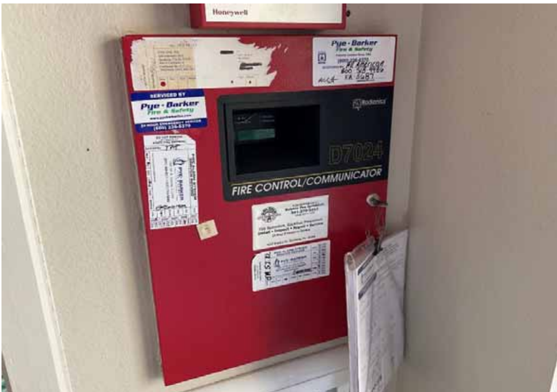
Pavilion Clubhouse Fire Alarm Panel
