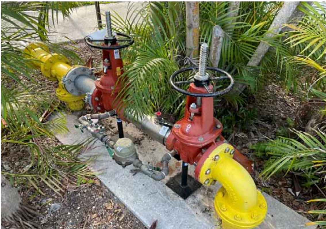
Backflow Preventer - Pavilion Clubhouse
