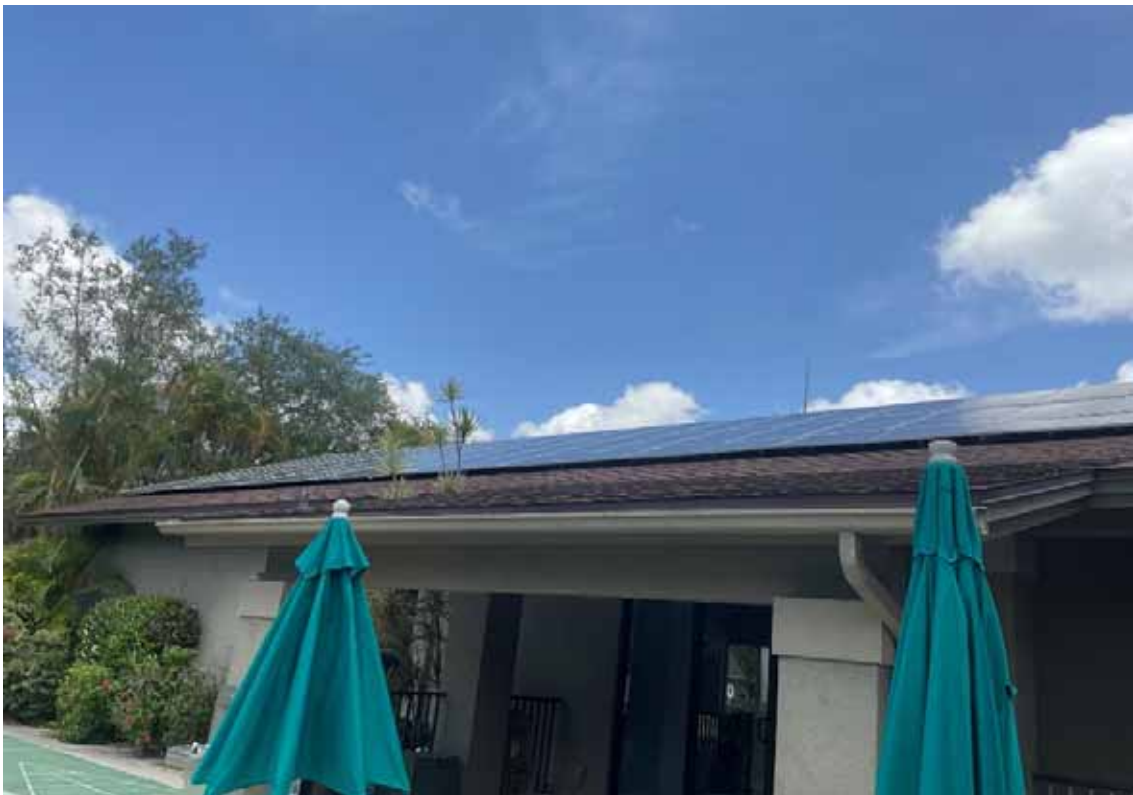
Pavilion Clubhouse Solar Array
