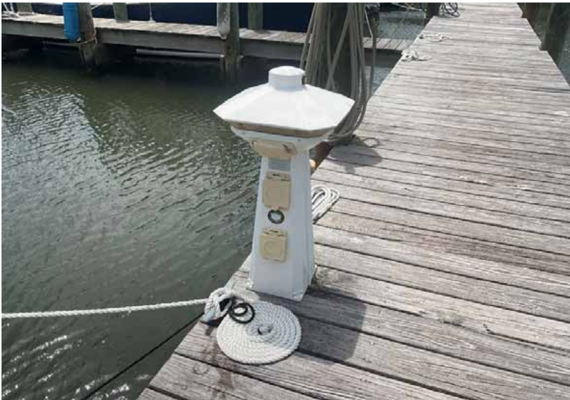
Harbor Marina Power Pedestal
