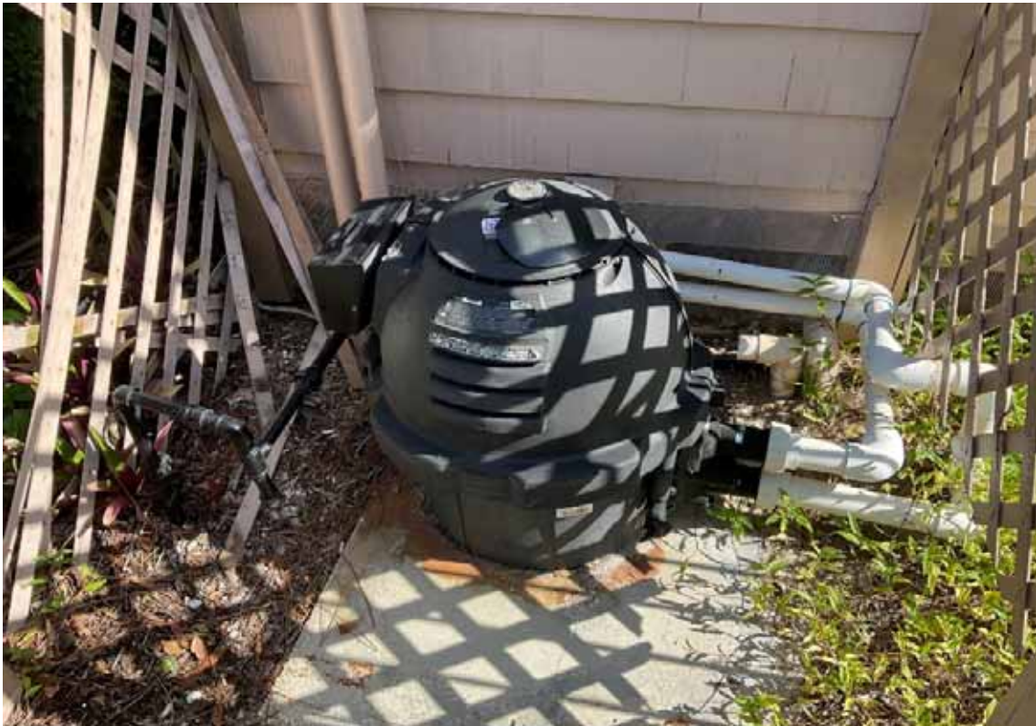
Glenhouse Pool Equipment, Heater
