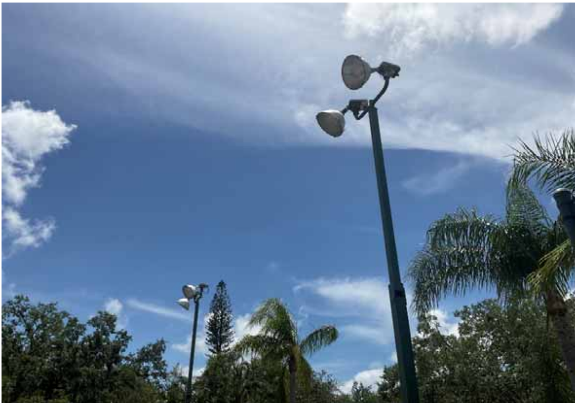
Harbor Club Tennis Court Lighting
