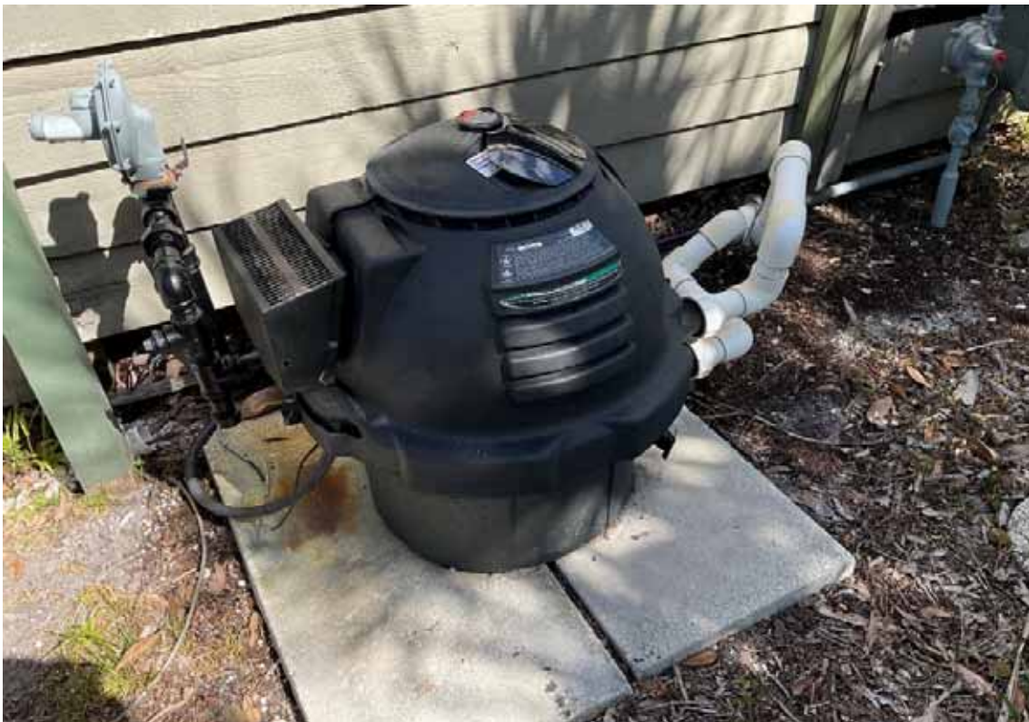
Wilbanks Pool Equipment, Heater
