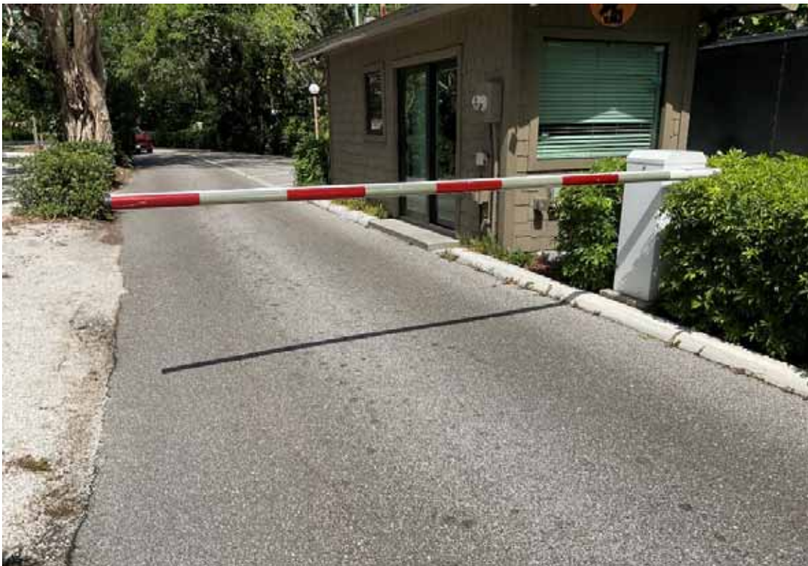
Gate Operator, Barrier - Exit
