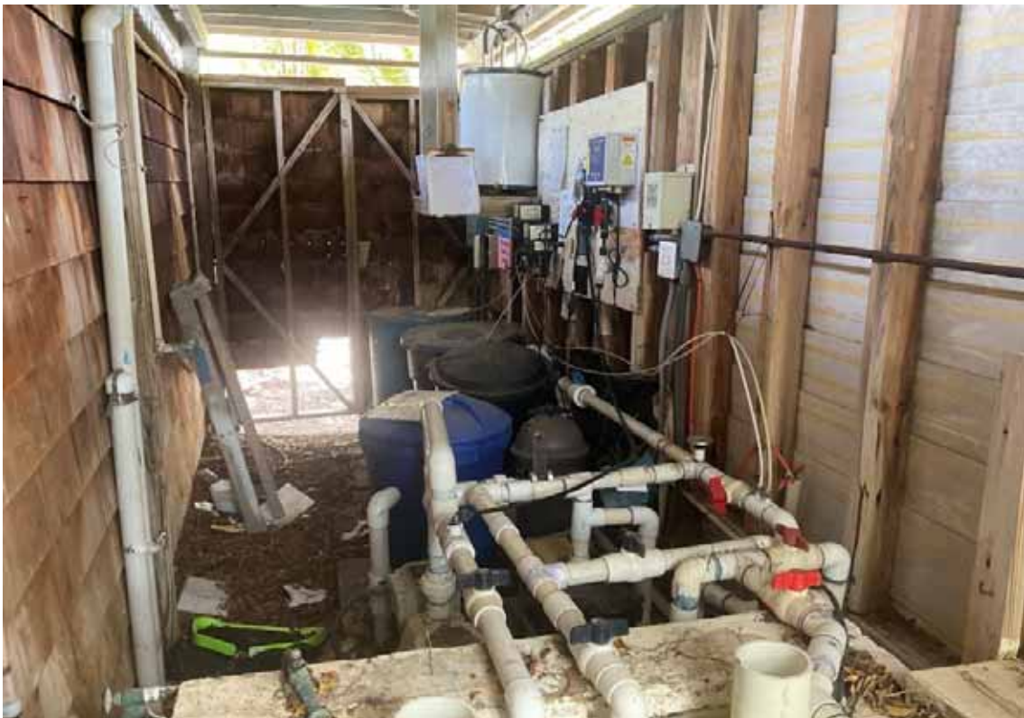
Far Harbor Pool Equipment
