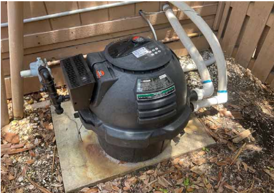
Brookhouse Pool Equipment, Heater
