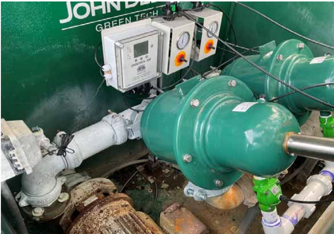
Booster Pump Station - Vamo Road
