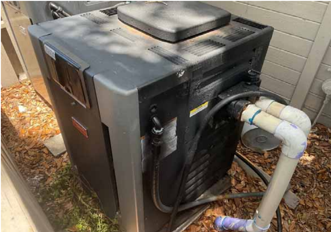
Harbor Club Spa Equipment, Heater
