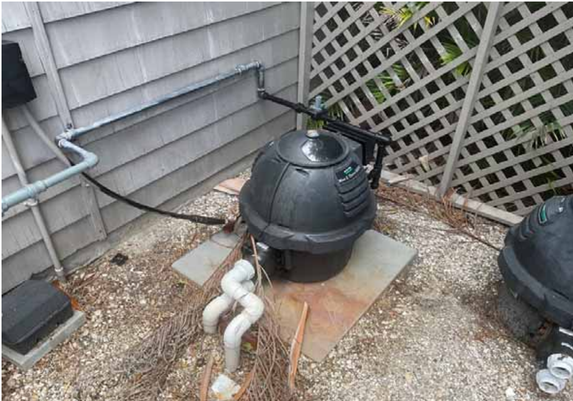
Far Harbor Pool Equipment, Heater
