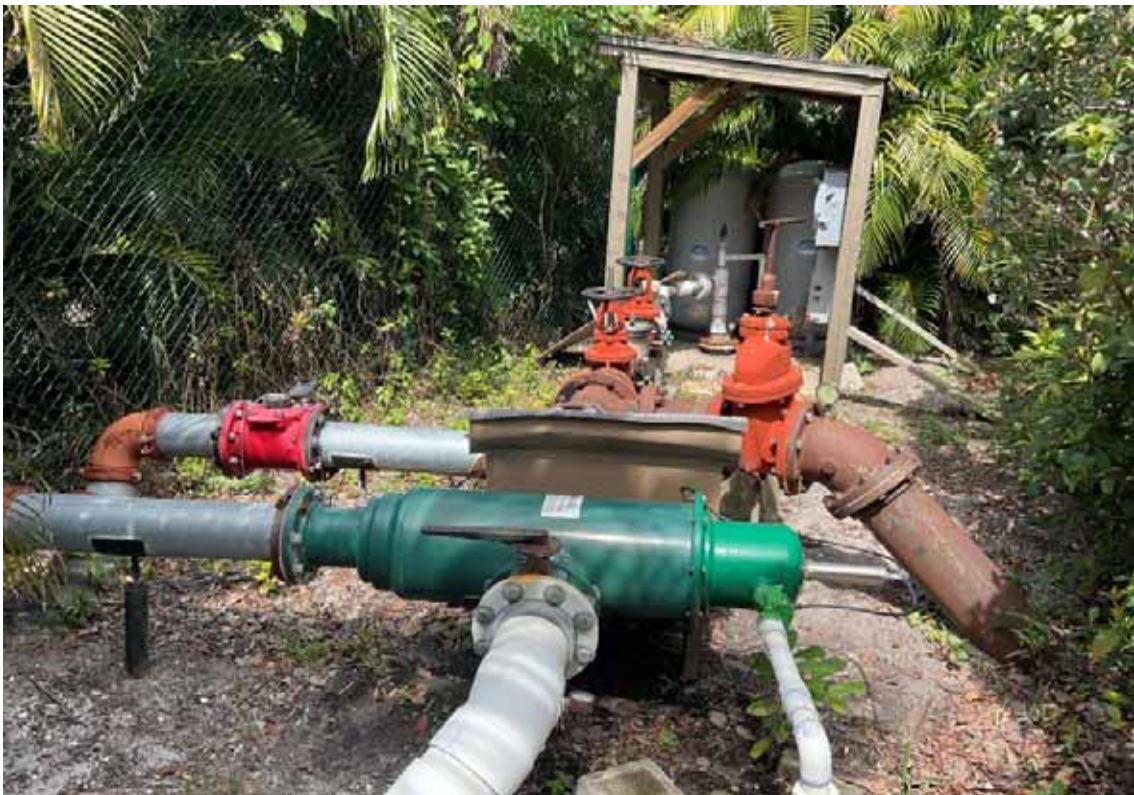
Well Pump - Treehouse
