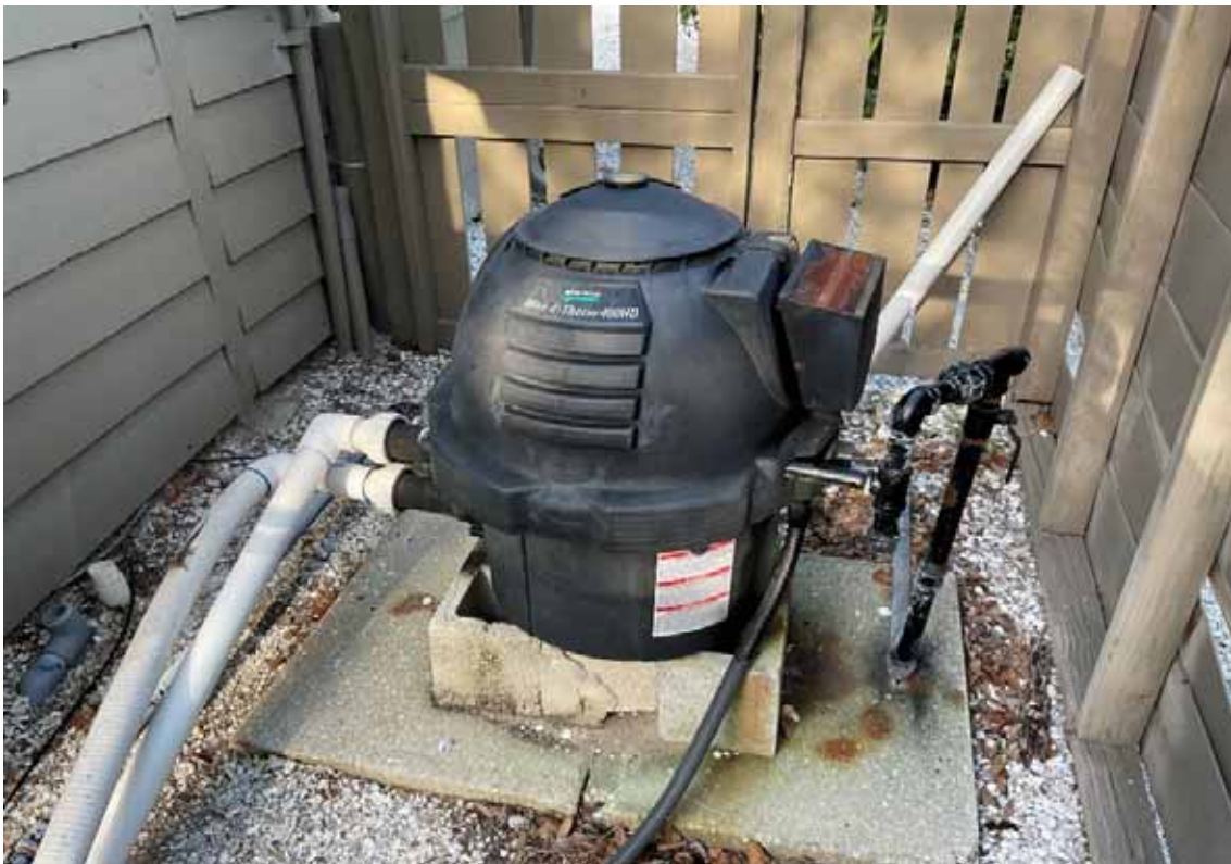
Pavilion Pool Equipment, Heater
