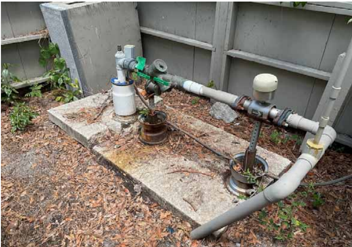
Well Pump - 4 Way
