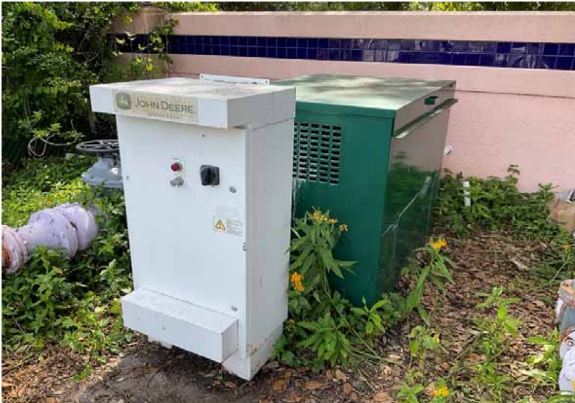
Booster Pump Station - Vamo Road
