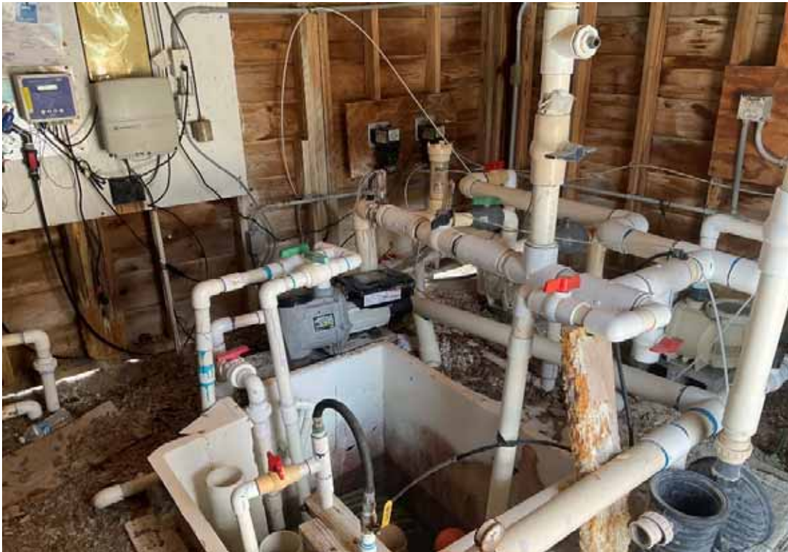
Pavilion Pool Equipment
