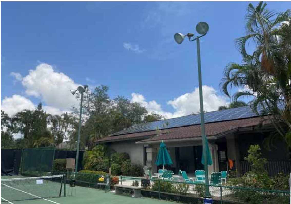
Pavilion Tennis Court Lighting
