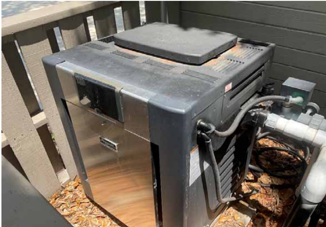
Harbor Club Pool Equipment, Heater
