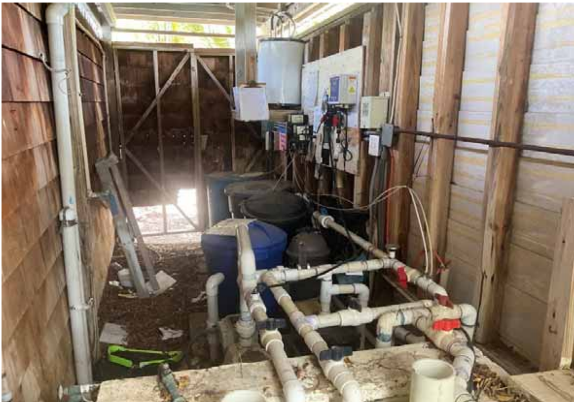
Far Harbor Pool Equipment
