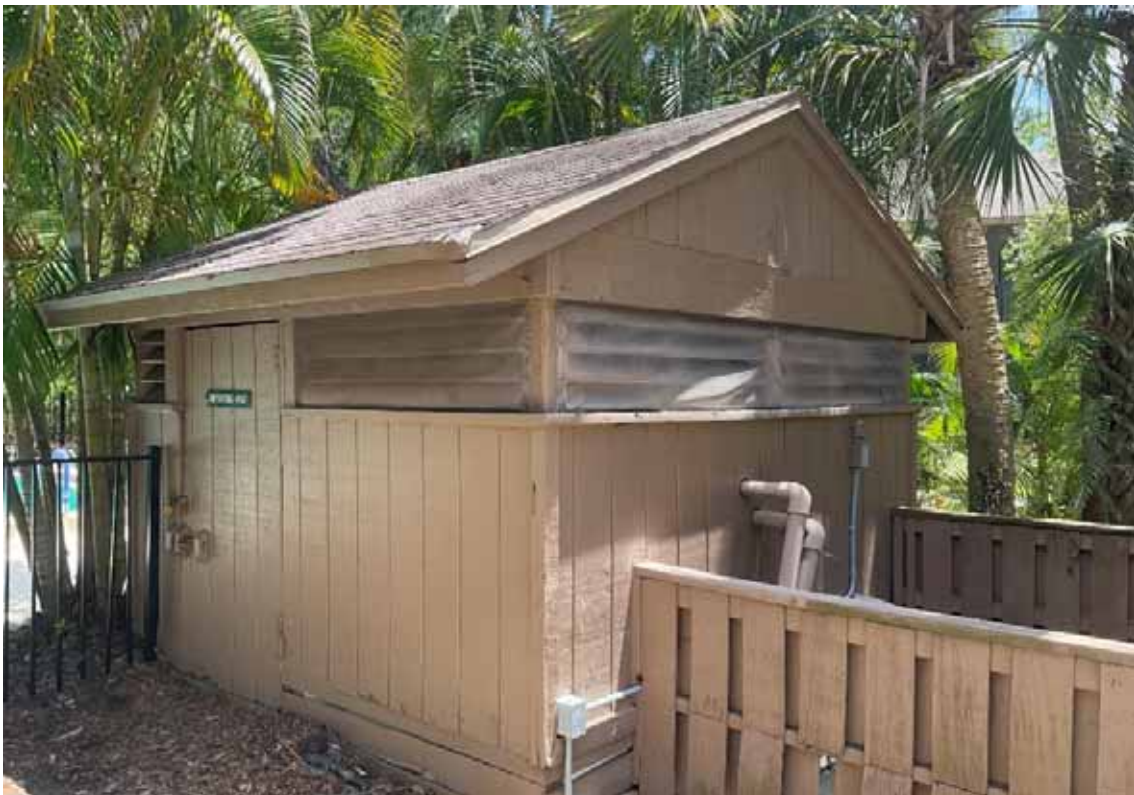
Brookhouse Pool Equipment Bldg
