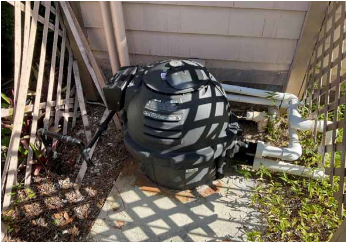
Glenhouse Pool Equipment, Heater
