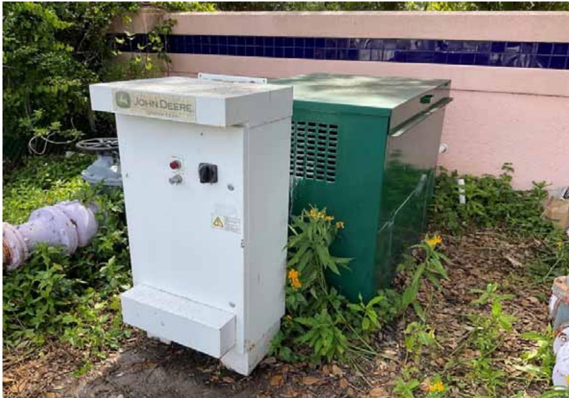
Booster Pump Station - Vamo Road
