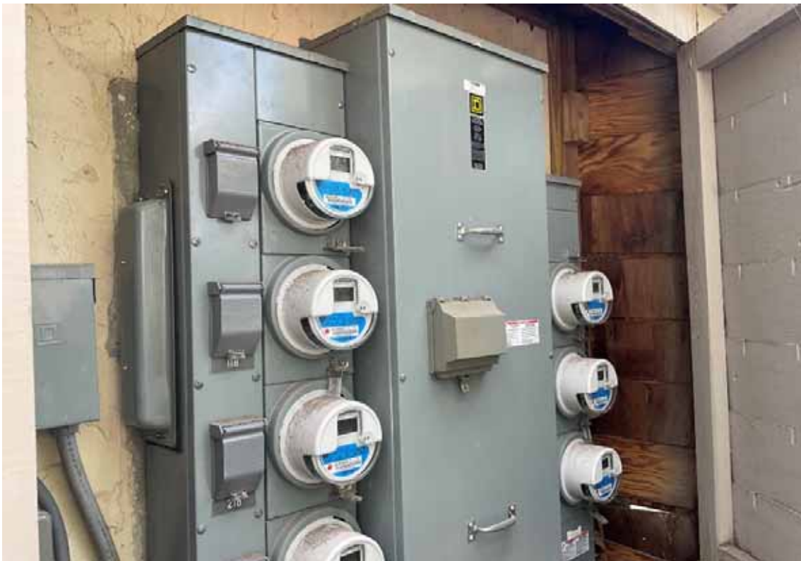
Condo Bldg Electrical Panel (New)
