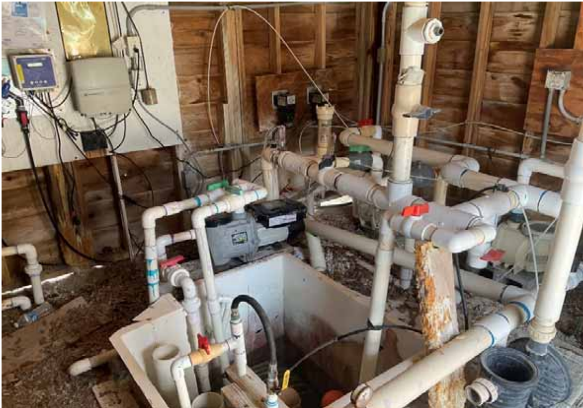
Pavilion Pool Equipment
