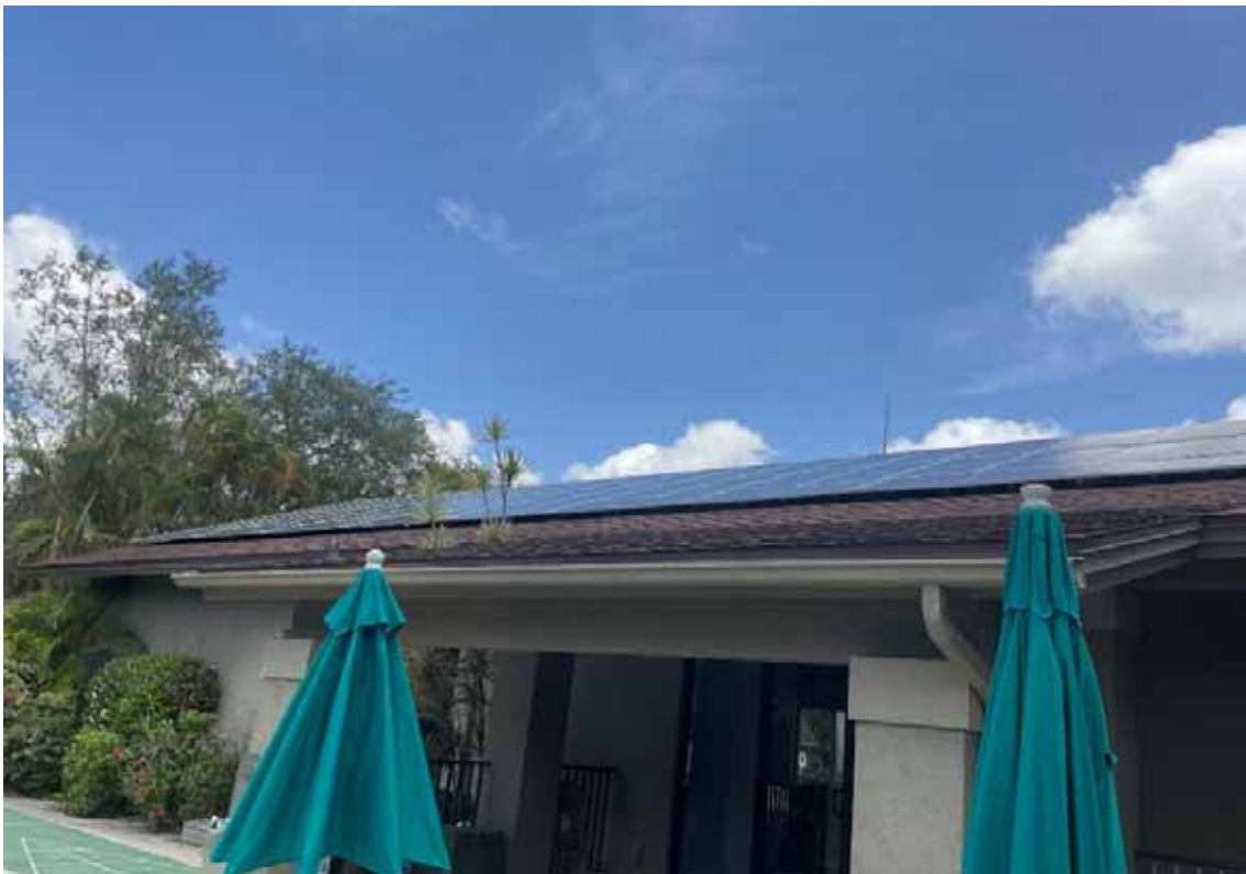
Pavilion Clubhouse Solar Array
