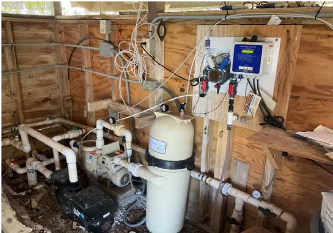
Harbor Club Spa Equipment
