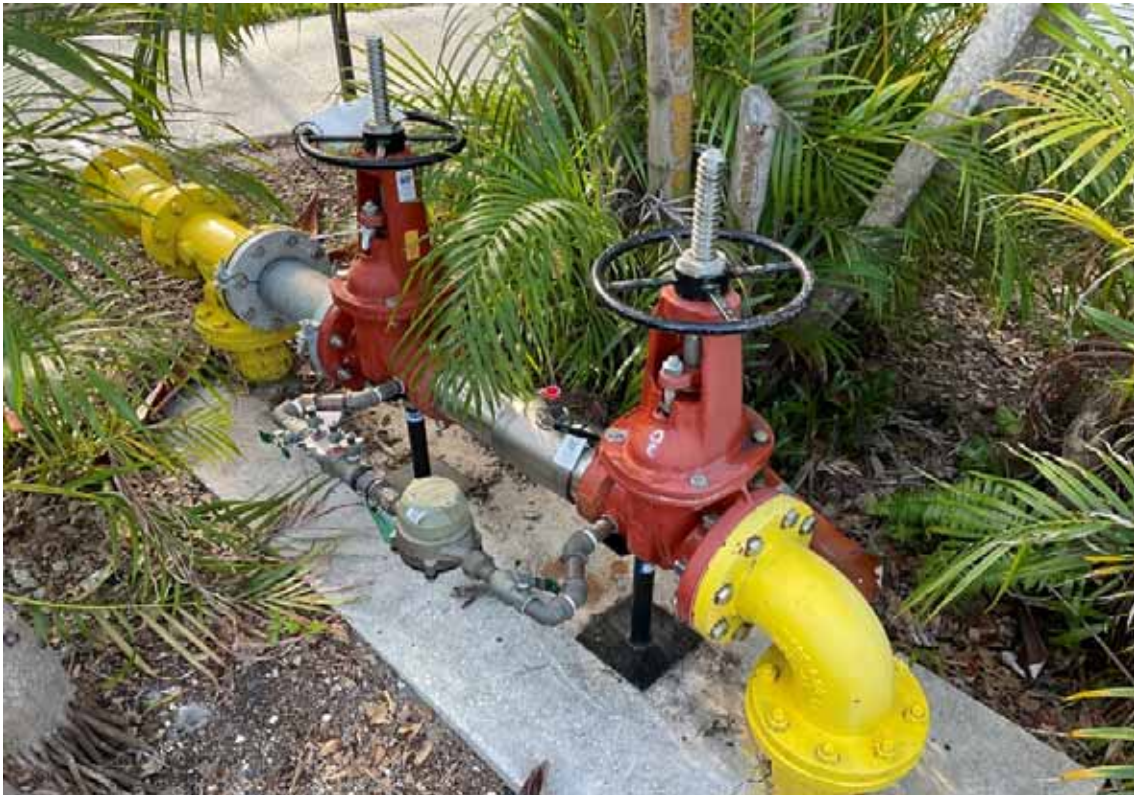
Backflow Preventer - Pavilion Clubhouse
