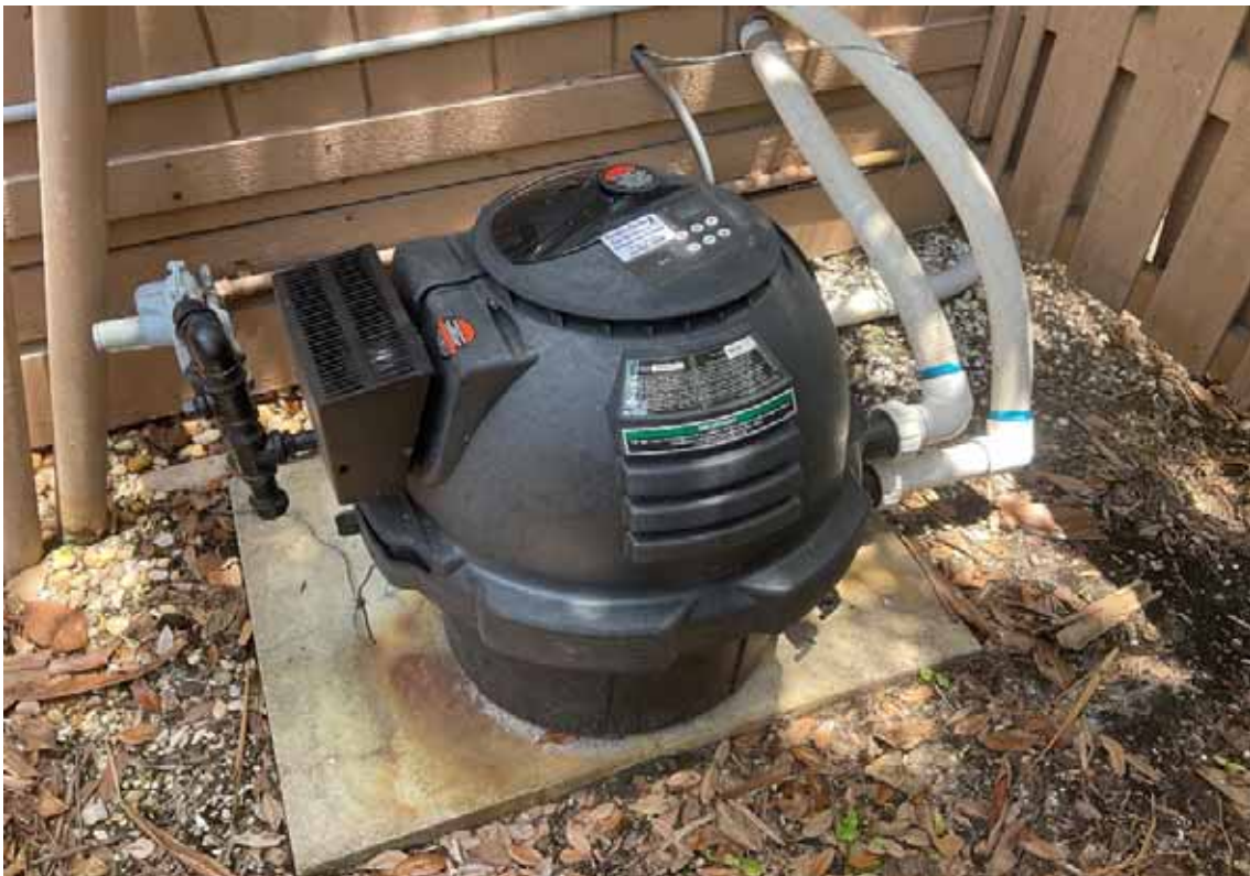
Brookhouse Pool Equipment, Heater
