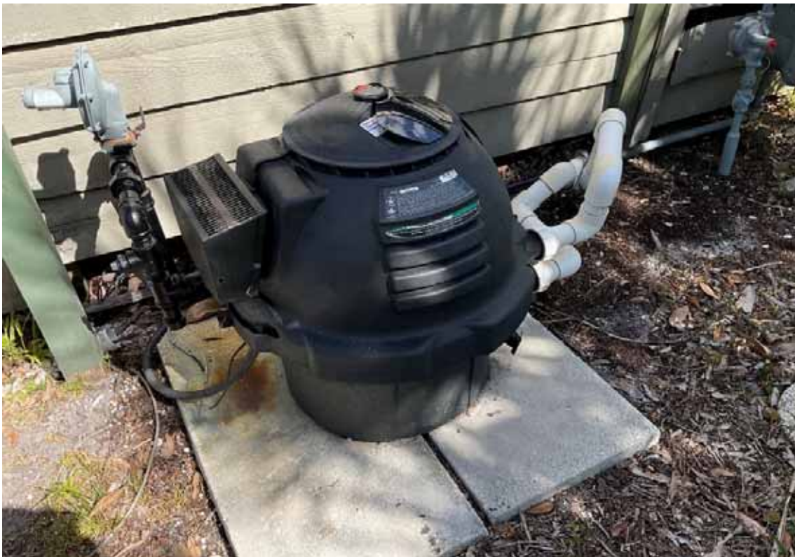
Wilbanks Pool Equipment, Heater
