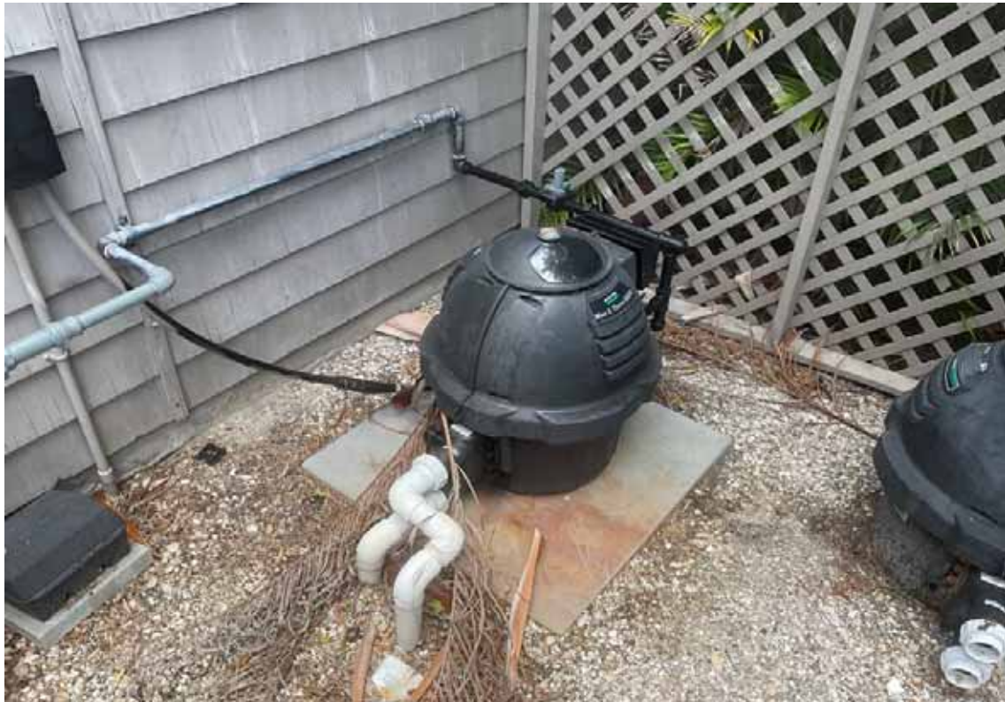
Far Harbor Pool Equipment, Heater
