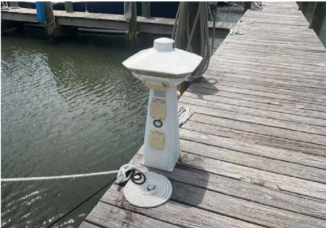
Harbor Marina Power Pedestal
