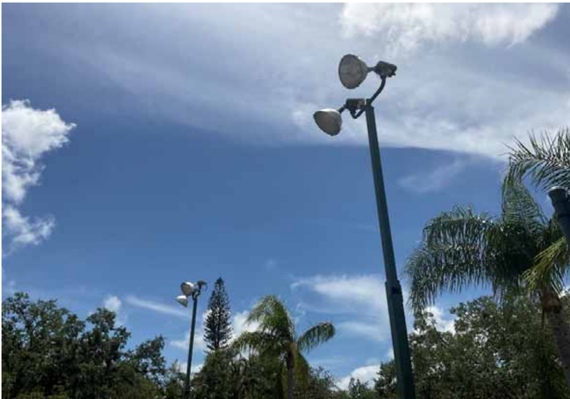
Harbor Club Tennis Court Lighting
