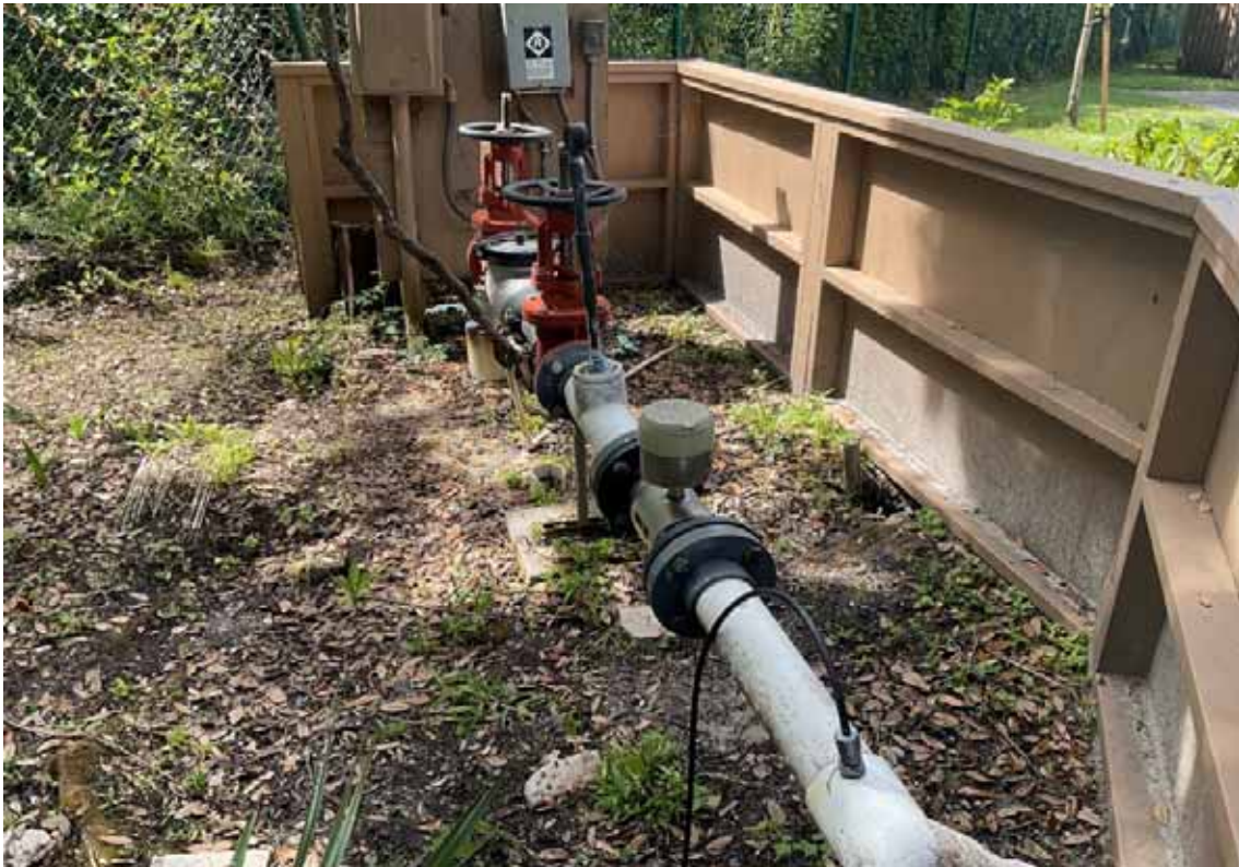
Well Pump - Brookhouse
