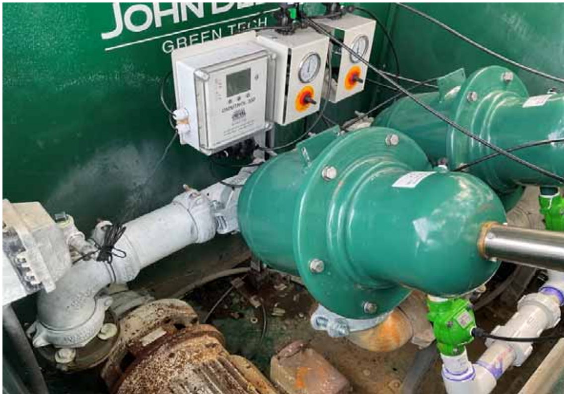
Booster Pump Station - Vamo Road
