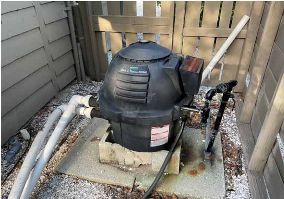
Pavilion Pool Equipment, Heater
