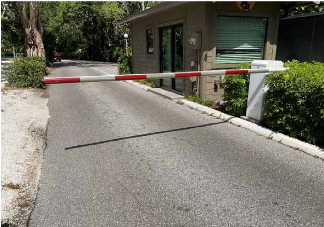
Gate Operator, Barrier - Exit
