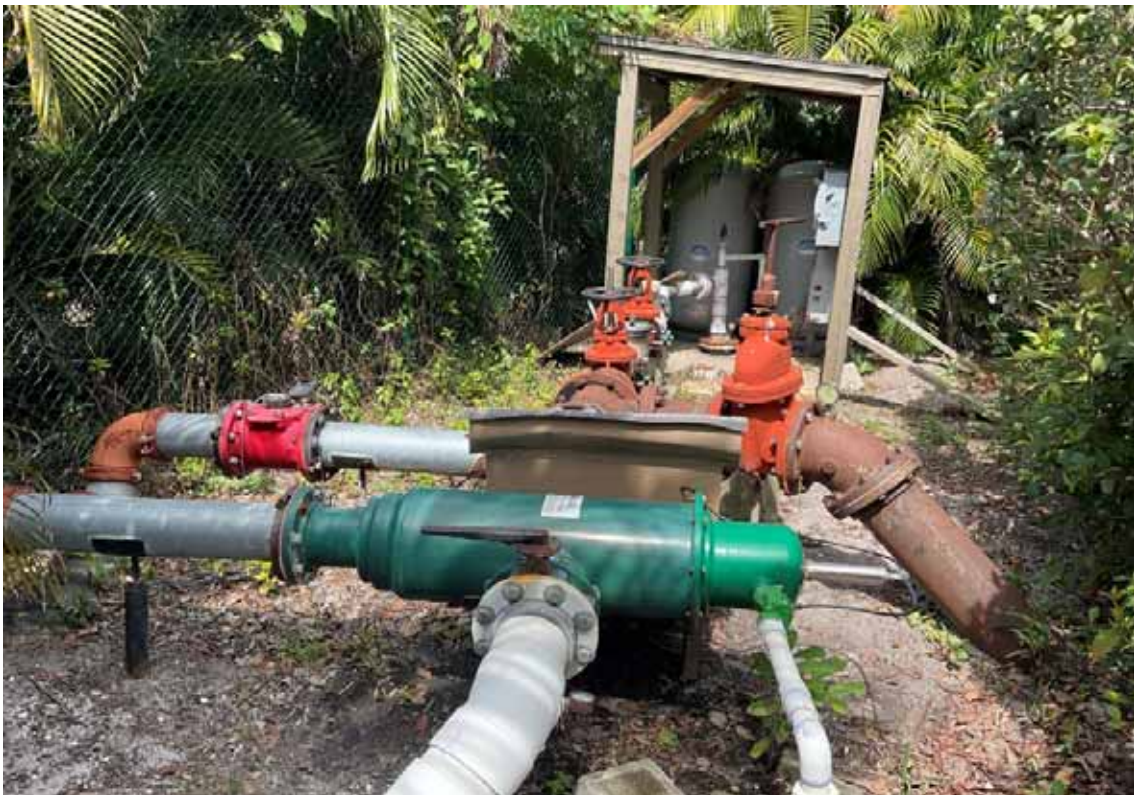
Well Pump - Treehouse
