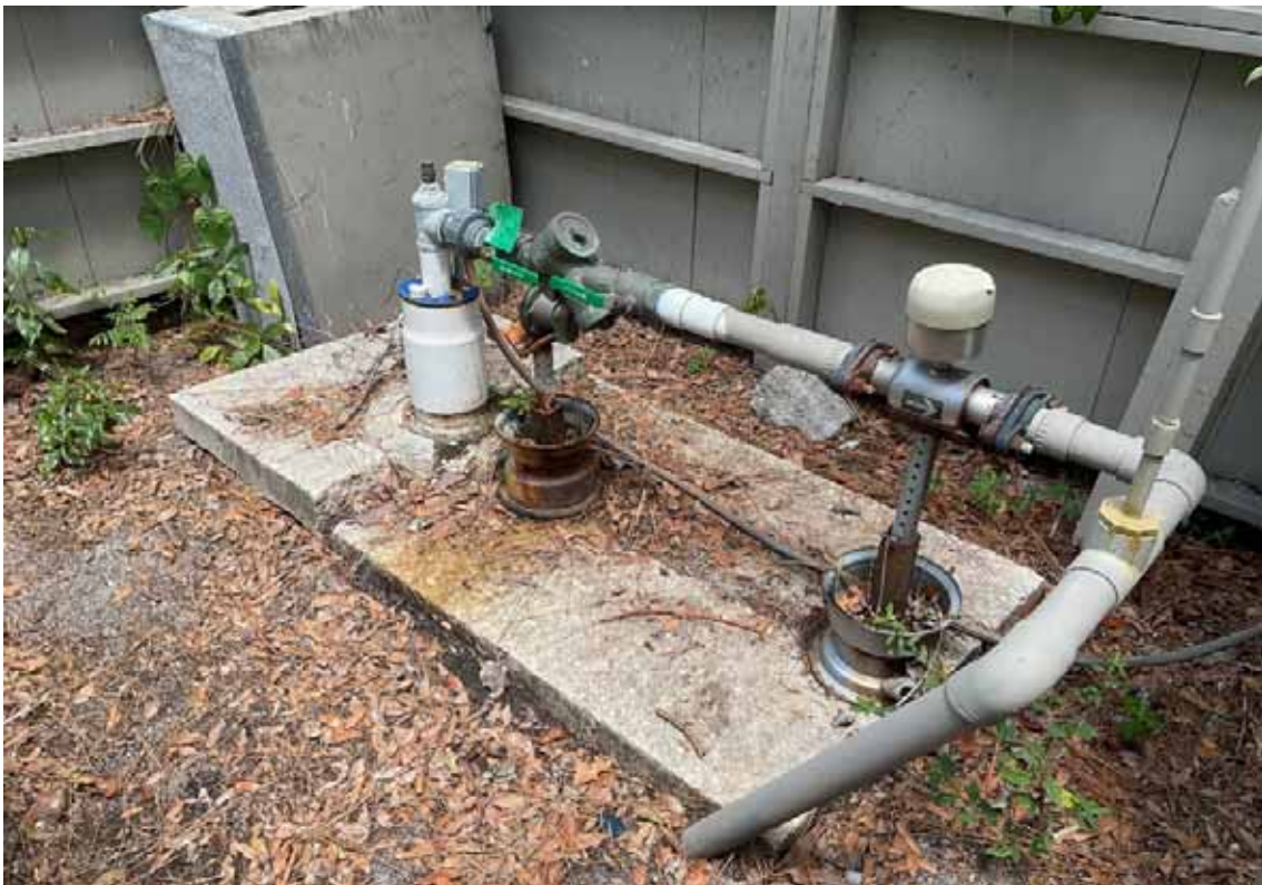
Well Pump - 4 Way
