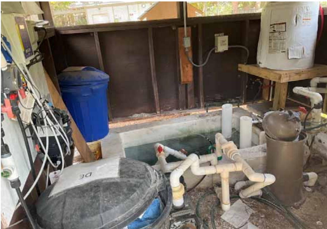
Glenhouse Pool Equipment
