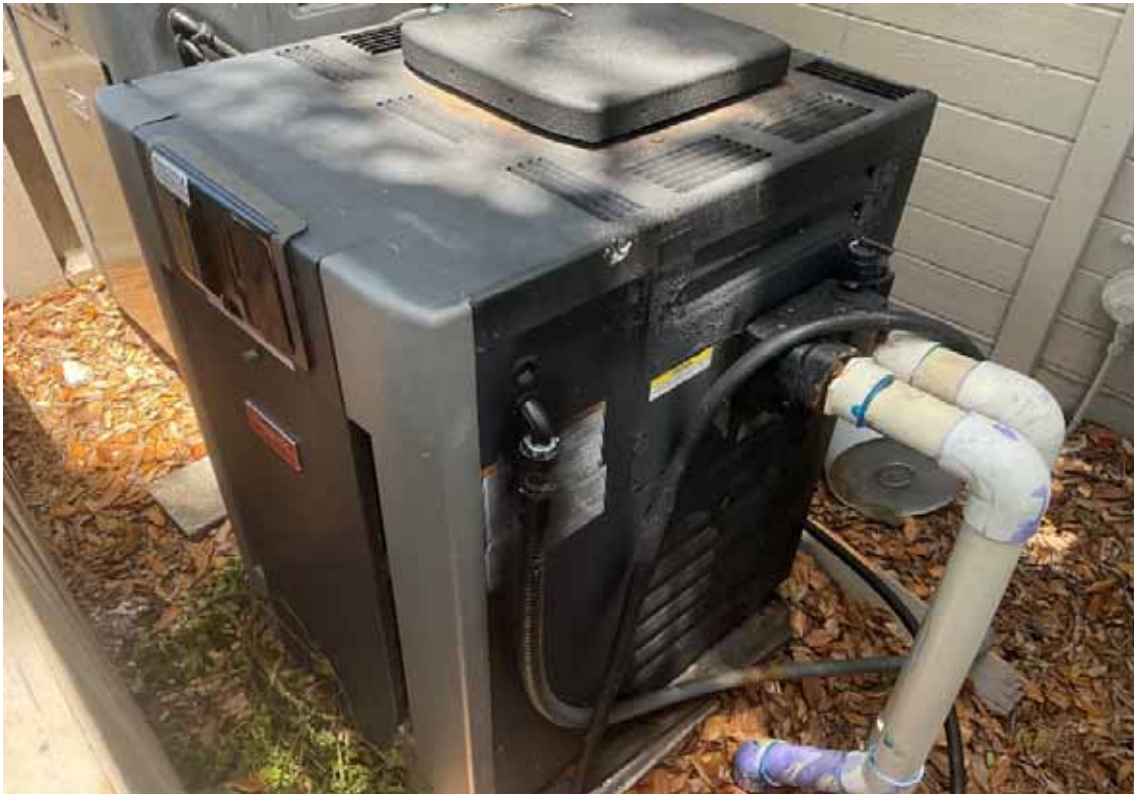
Harbor Club Spa Equipment, Heater
