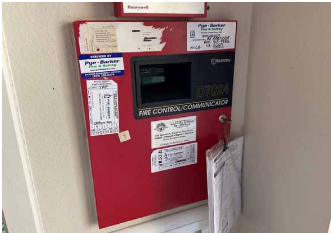
Pavilion Clubhouse Fire Alarm Panel
