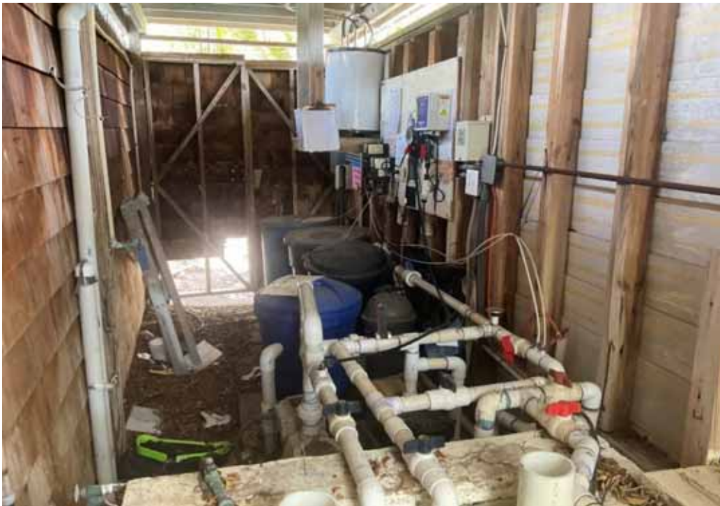
Far Harbor Pool Equipment
