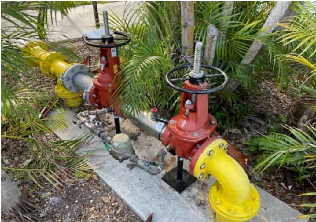
Backflow Preventer - Pavilion Clubhouse
