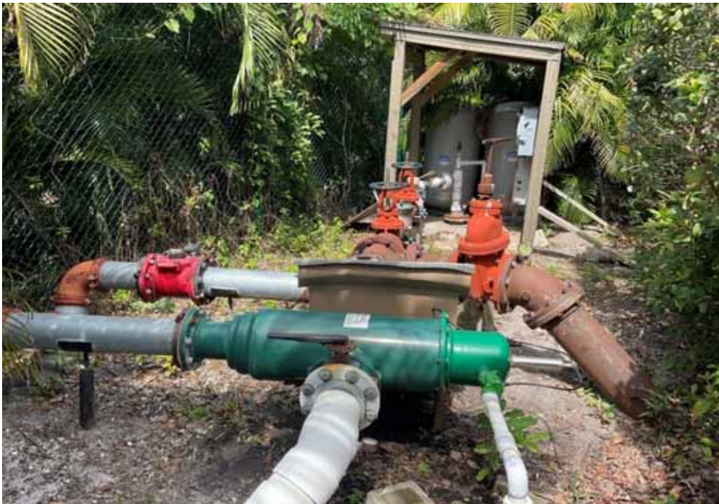
Well Pump - Treehouse
