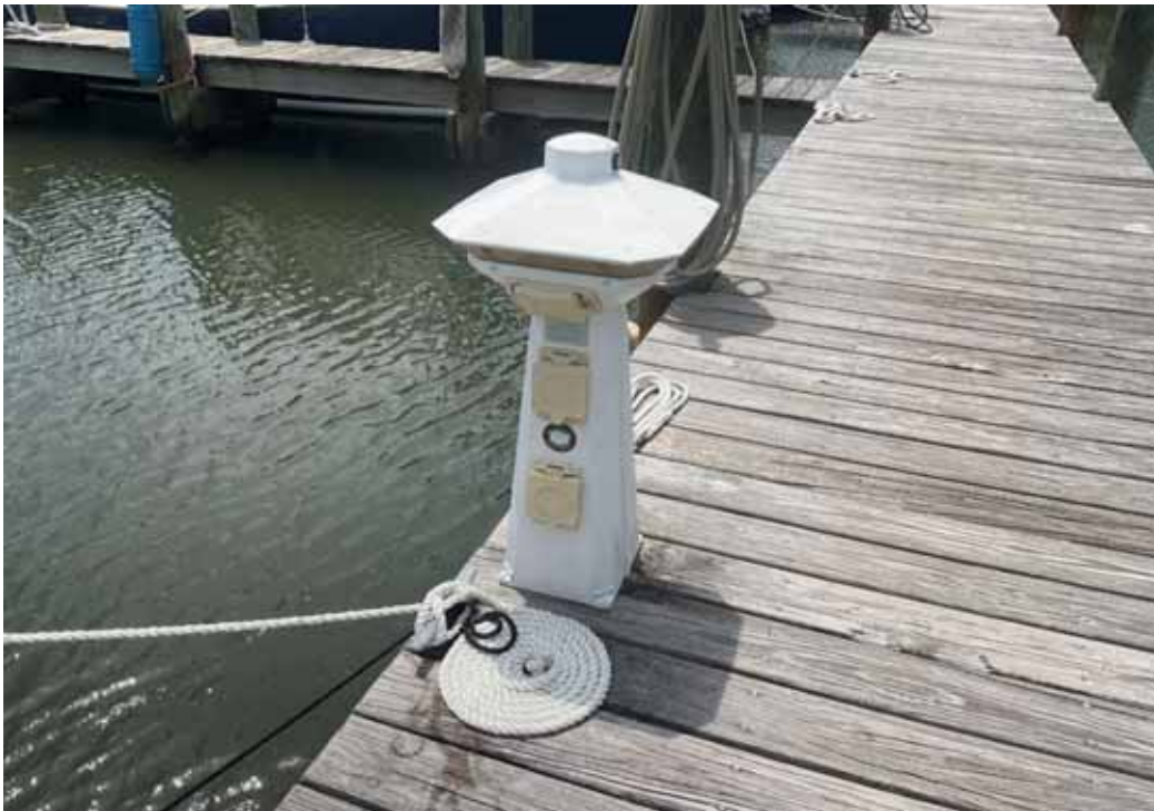
Harbor Marina Power Pedestal
