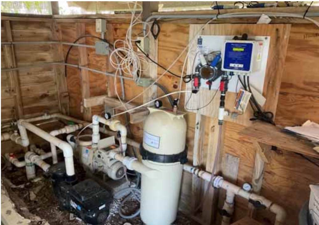
Harbor Club Spa Equipment
