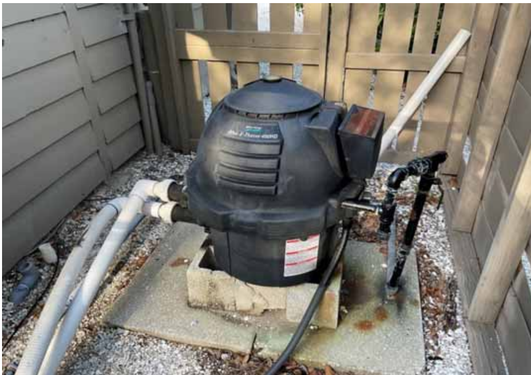
Pavilion Pool Equipment, Heater
