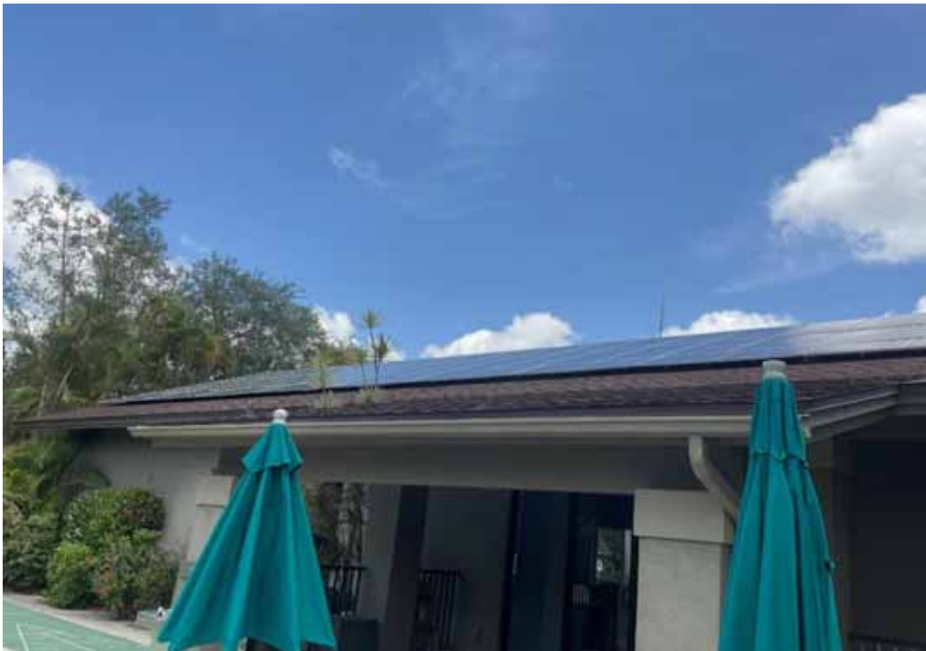
Pavilion Clubhouse Solar Array
