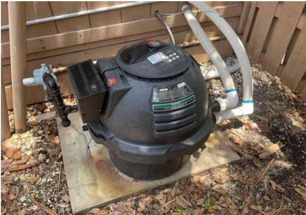
Brookhouse Pool Equipment, Heater
