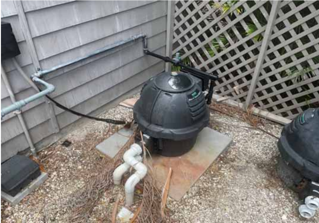
Far Harbor Pool Equipment, Heater
