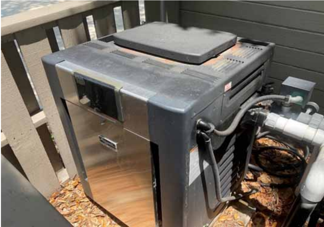
Harbor Club Pool Equipment, Heater
