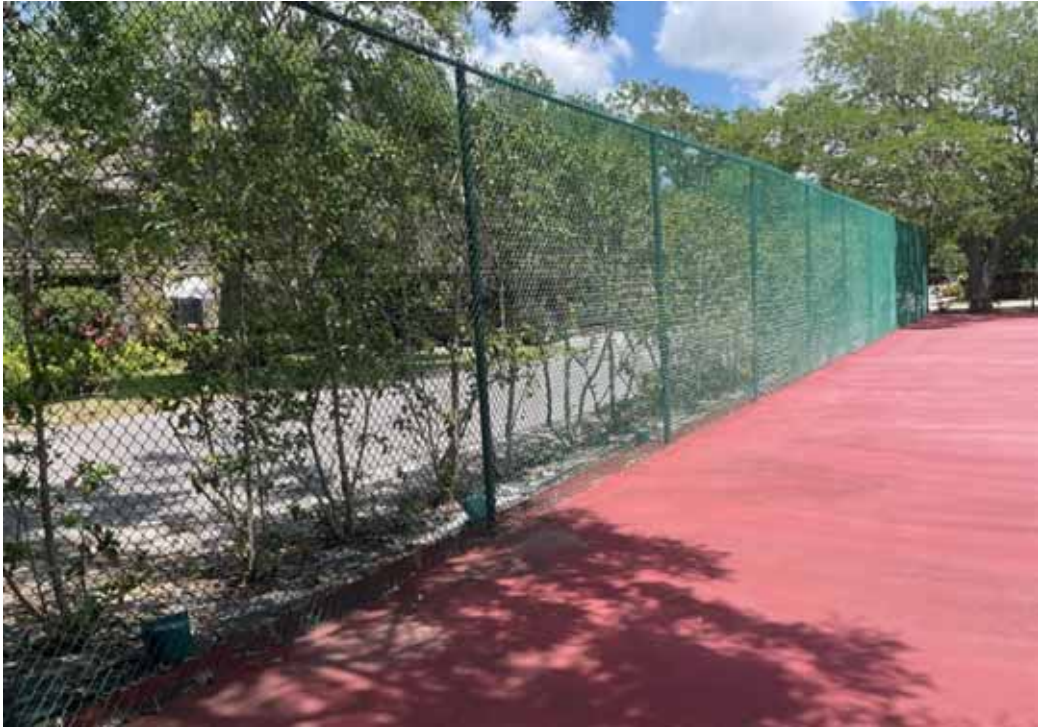
Harbor Club Tennis Court Fence
