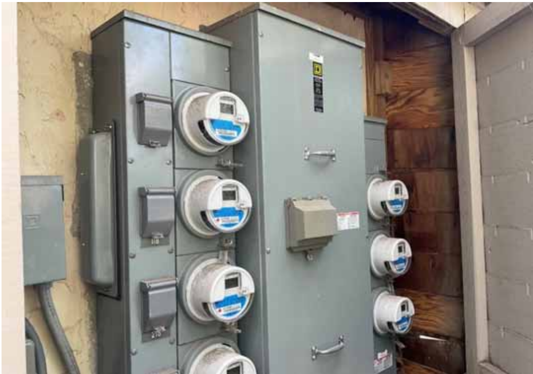
Condo Bldg Electrical Panel (New)
