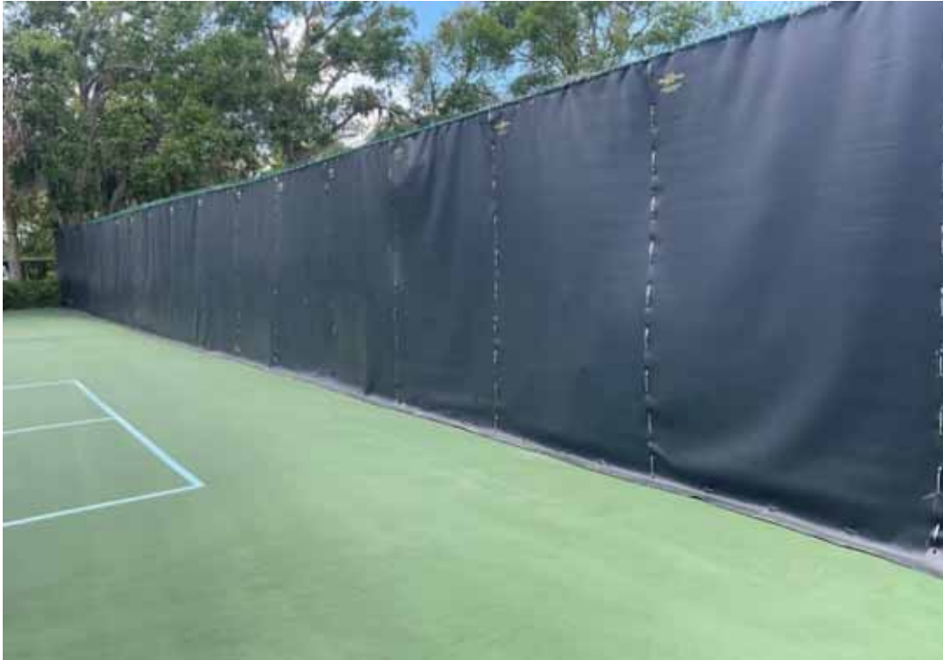
Pavilion Tennis Court Acoustifence Panels
