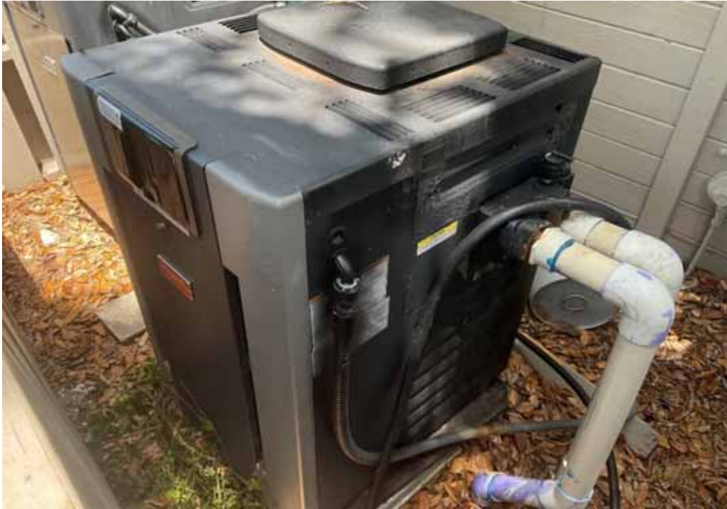
Harbor Club Spa Equipment, Heater
