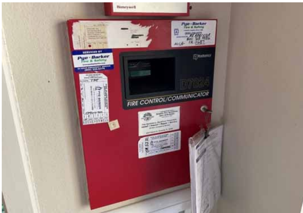
Pavilion Clubhouse Fire Alarm Panel
