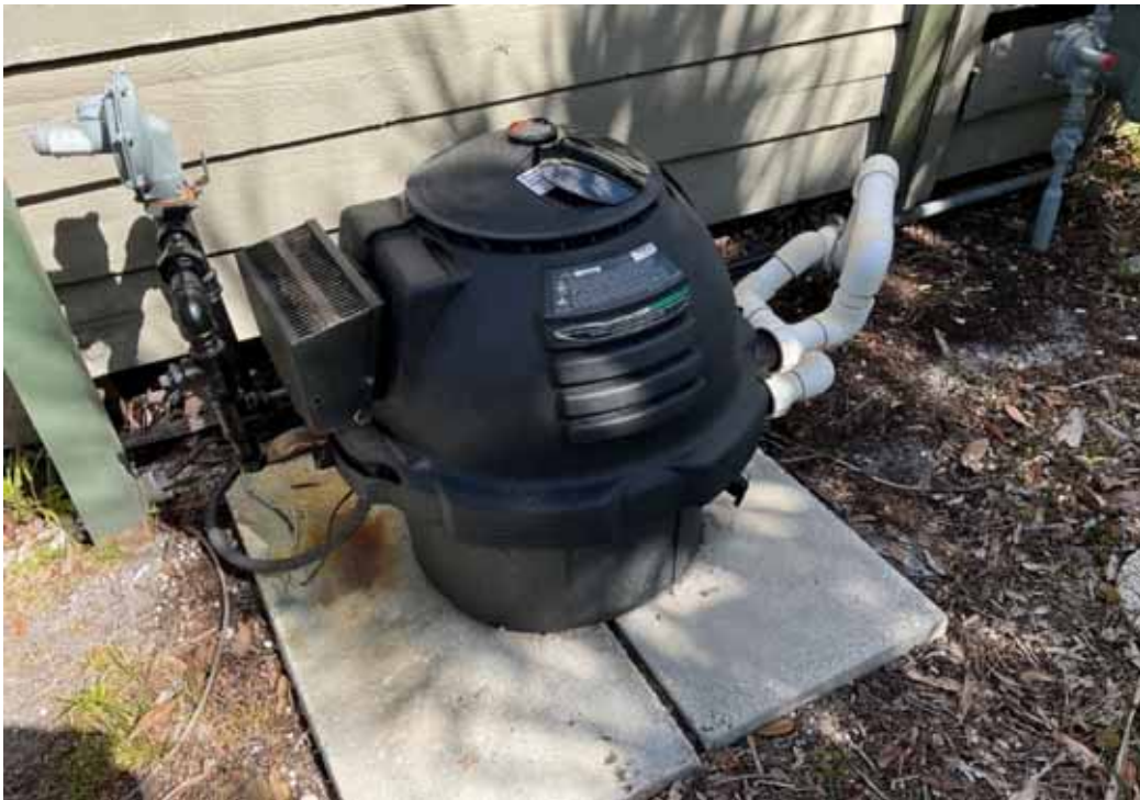
Wilbanks Pool Equipment, Heater
