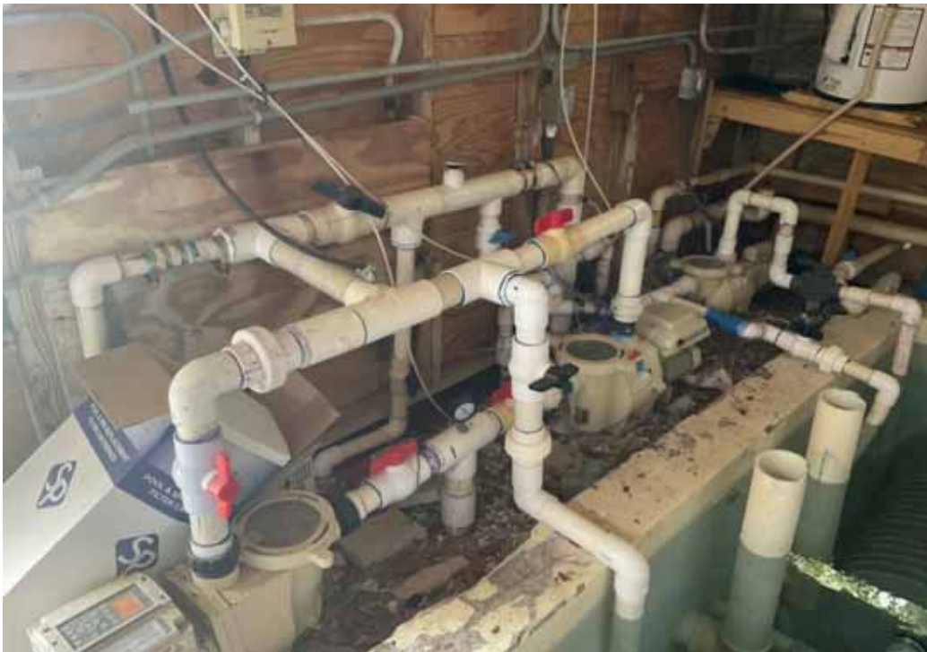
Harbor Club Pool Equipment
