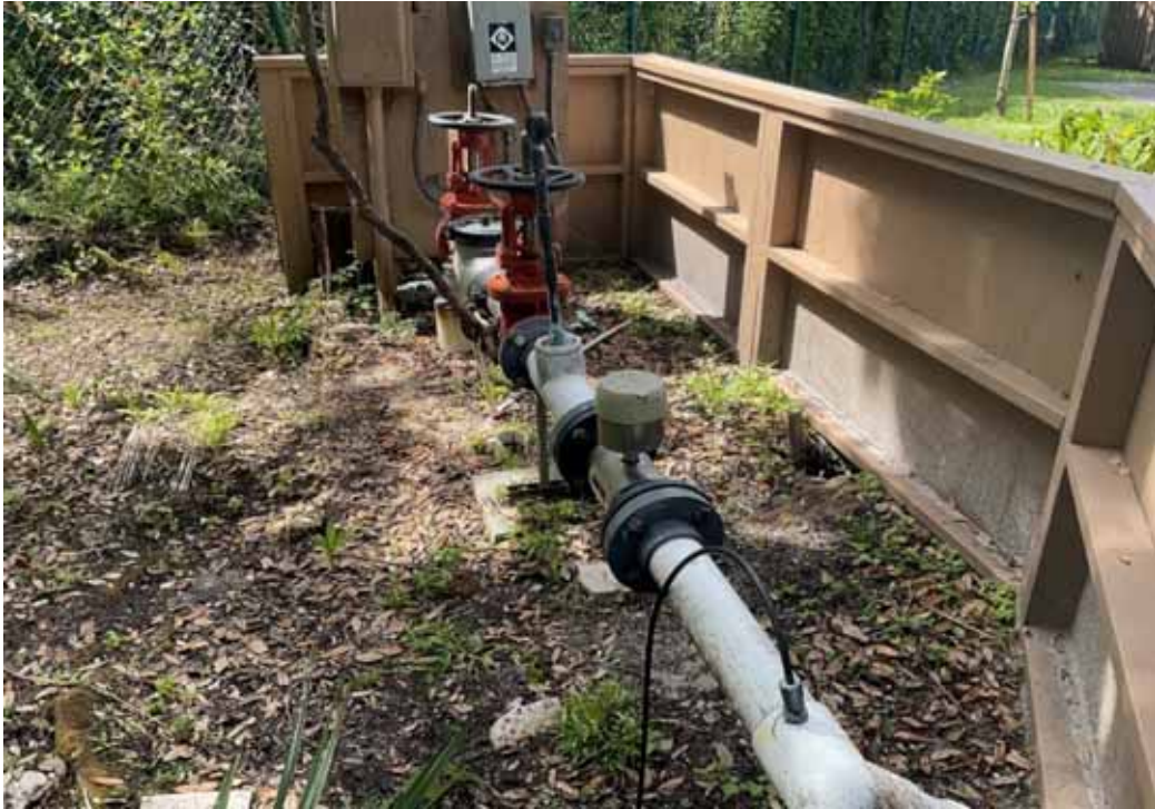
Well Pump - Brookhouse
