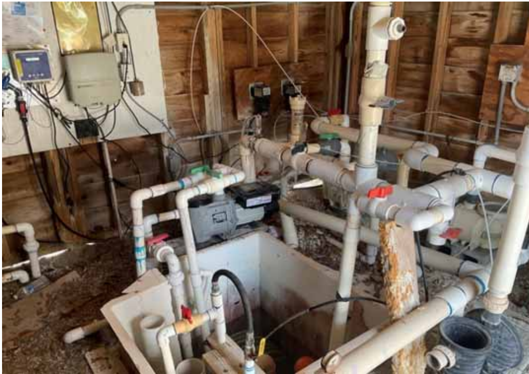
Pavilion Pool Equipment
