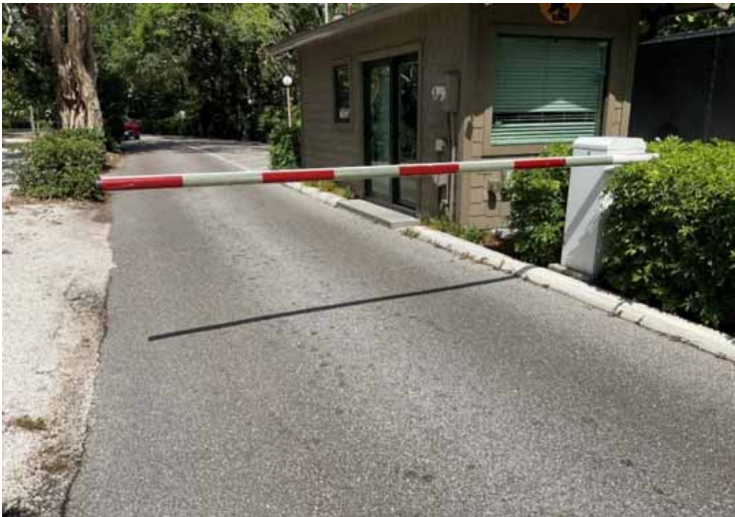
Gate Operator, Barrier - Exit
